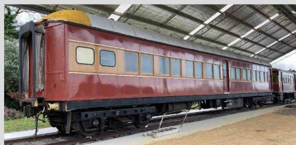
▲ ACT Rail Holdings received a grant for the replacement of the roof covering for FS 2023.
